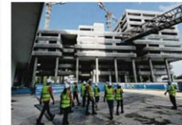
The SIT campus is expected to be operational by the second half of 2024. ST PHOTO: SHINTARO TAY
