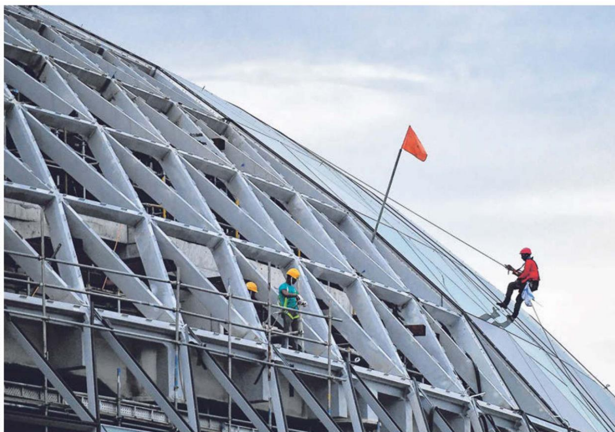
Foreign workers at Jewel Changi Airport when it was under construction in 2017. A big part of Singapore's national identity is in the skyline, attached to our architectural icons, buildings and infrastructure, say the writers, who point out that dominant narratives of the Singapore story have often left out the low-wage migrant workers who build, clean, maintain and renovate the icons of our national pride. ST FILE PHOTO
