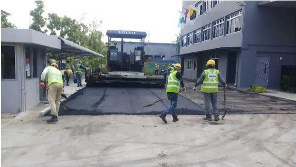
A road being laid with Magorium's product at a factory site in Tuas. (Photo: Magorium)
