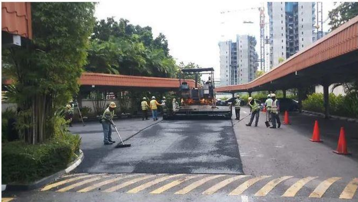
Earlier this month, the start-up's product was also used for road laying at a condominium in Marymount. (Photo: Magorium)
