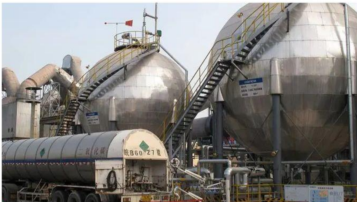
Carbon dioxide storage tanks are seen at a cement plant and carbon capture facility in Anhui province, China on Sep 11, 2019. (Photo: REUTERS/David Stanway)
