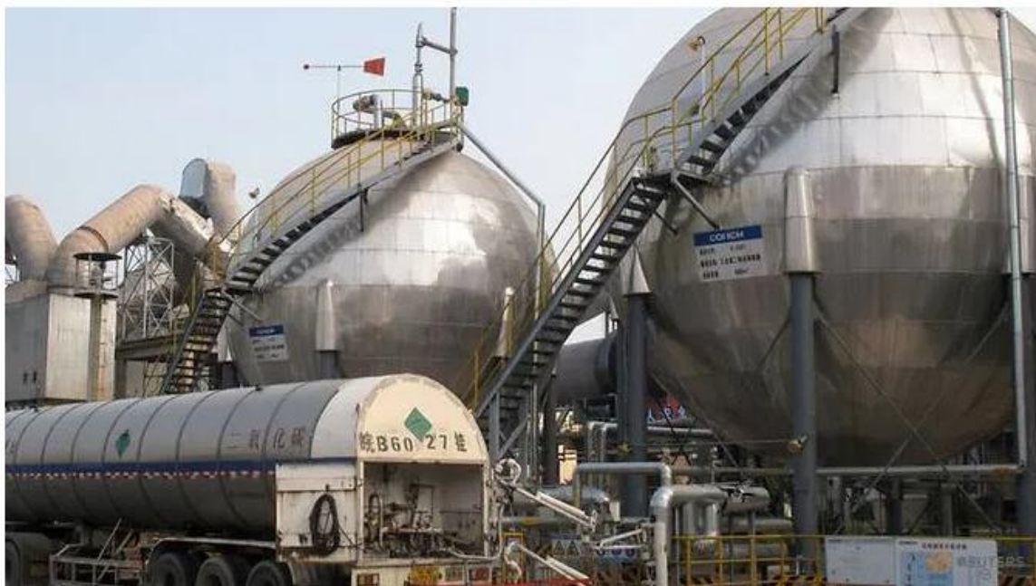
Carbon dioxide storage tanks are seen at a cement plant and carbon capture facility in Anhui province, China on Sep 11, 2019. (Photo: REUTERS/David Stanway)
