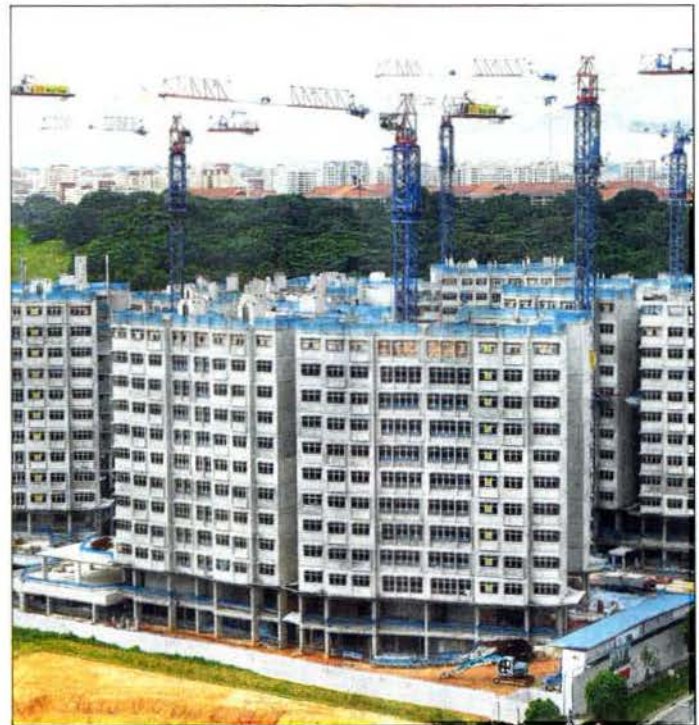
Build-To-Order flats at Fernvale Link. Providing additional housing grants is an acknowledgement that housing prices have run ahead of wage growth, particularly for the lower income group. ST PHOTO: SEAH KWANG PENG
