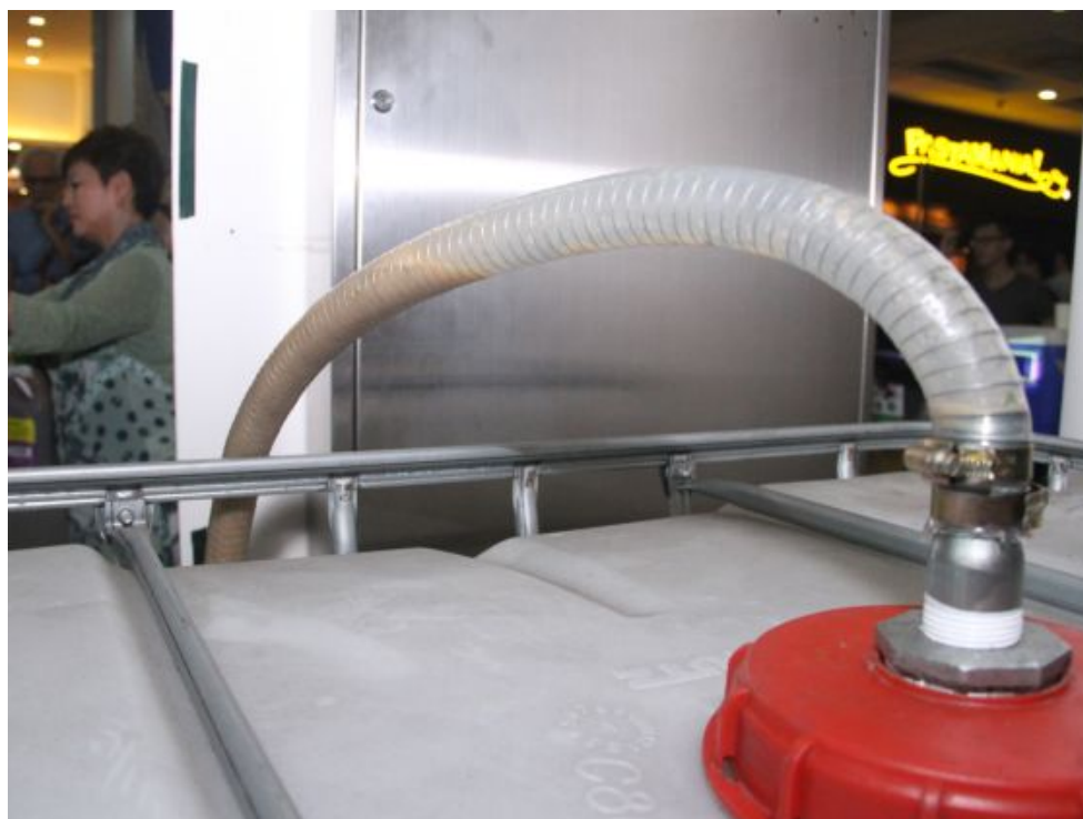
Food waste being pumped from the Bio-Regen unit into a large tank...
