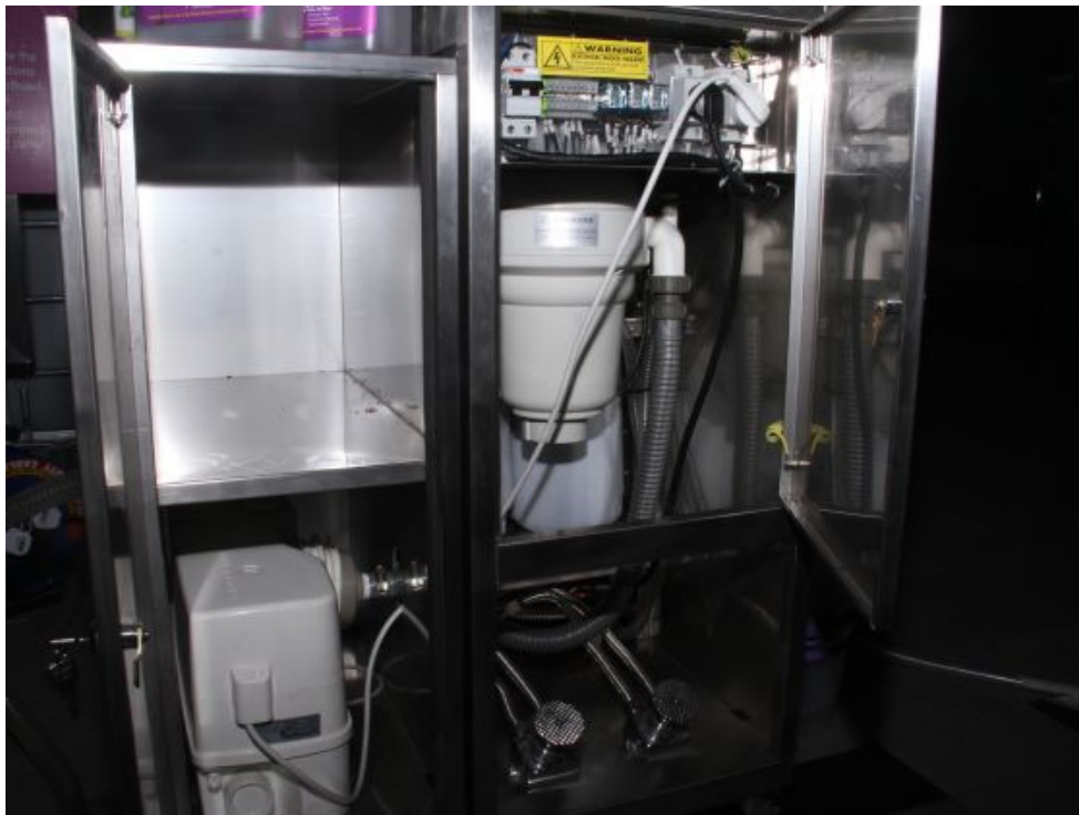
The insides of the Bio-Regen unit. Photo: Daryl Kang
