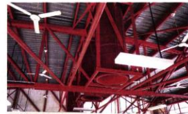
Specially developed for tropical climate, solar chimneys are made of metal that absorbs solar radiation. Placed on top of the roof or up high in a non-air-conditioned room, they suck out warm air from the room. Through convection, cool air will then rush into the room.
